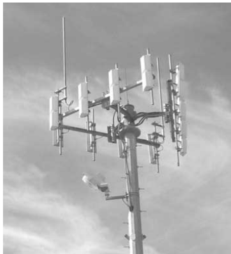
Figure 16.5 Sectorized base-station antenna.
