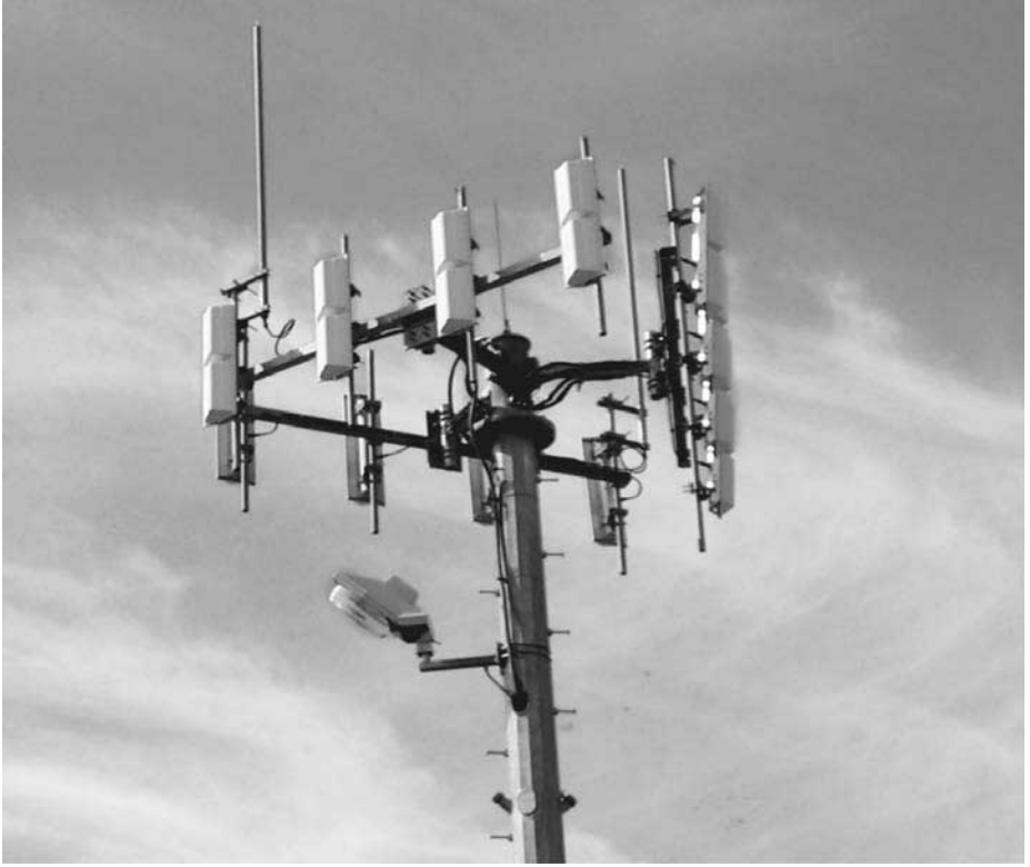
Figure 4.23 Triangular array of dipoles used as a sectoral base-station antenna for mobile communication.
